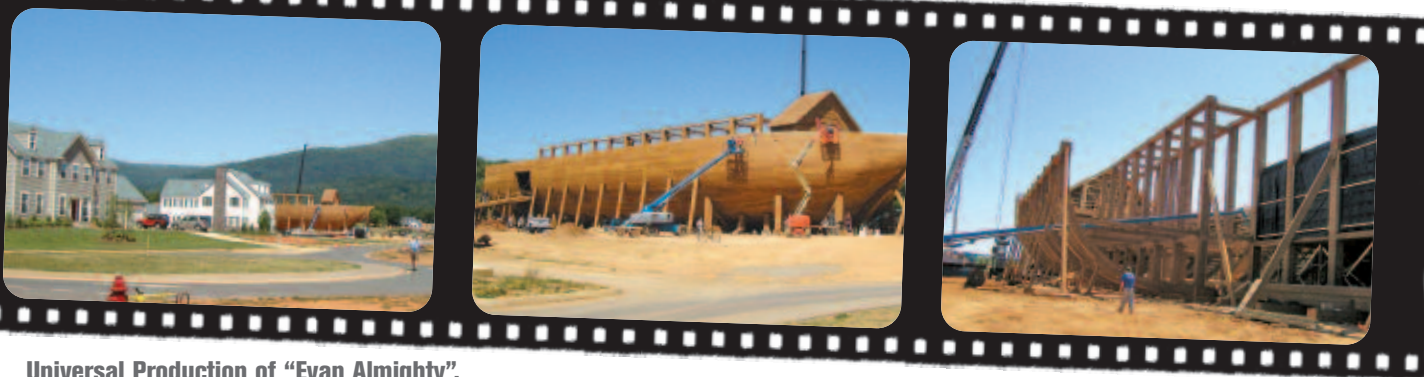
Universal Production of "Evan Almighty". It's Noah's Ark constructed in the jurisdiction of Local 487.
